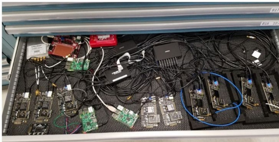
Figure 3-1 Wired RF devices in drawer with splitter and coax cable connectivity
