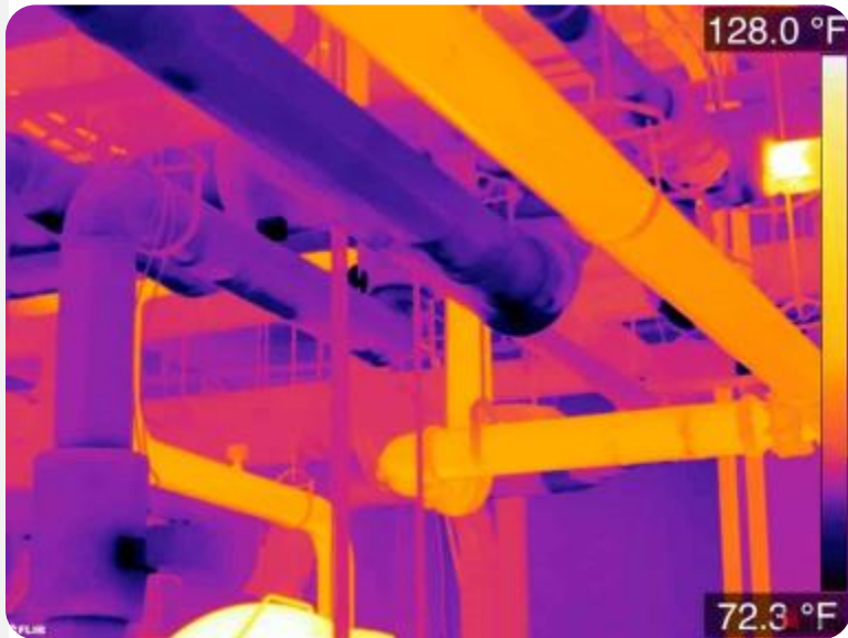
Hot Fluid Piping
